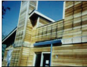
Iron stain on a building.
