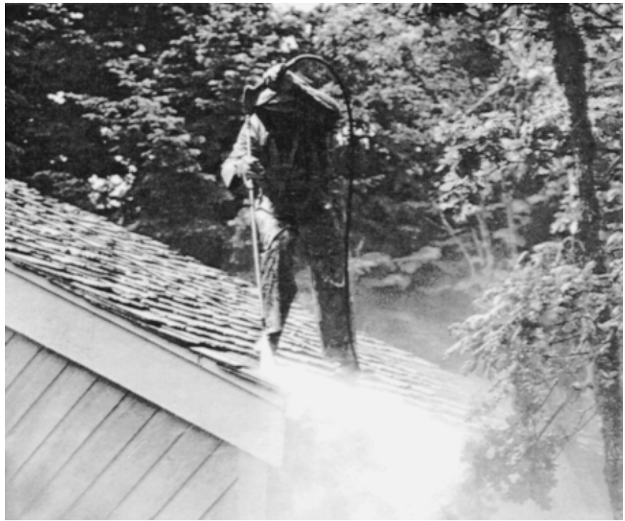
Figure 2.—High-pressure washers are effective in cleaning roof surfaces of debris and moss. Be careful when you use them in order to prevent unnecessary erosion of the shingle or shake surfaces.
