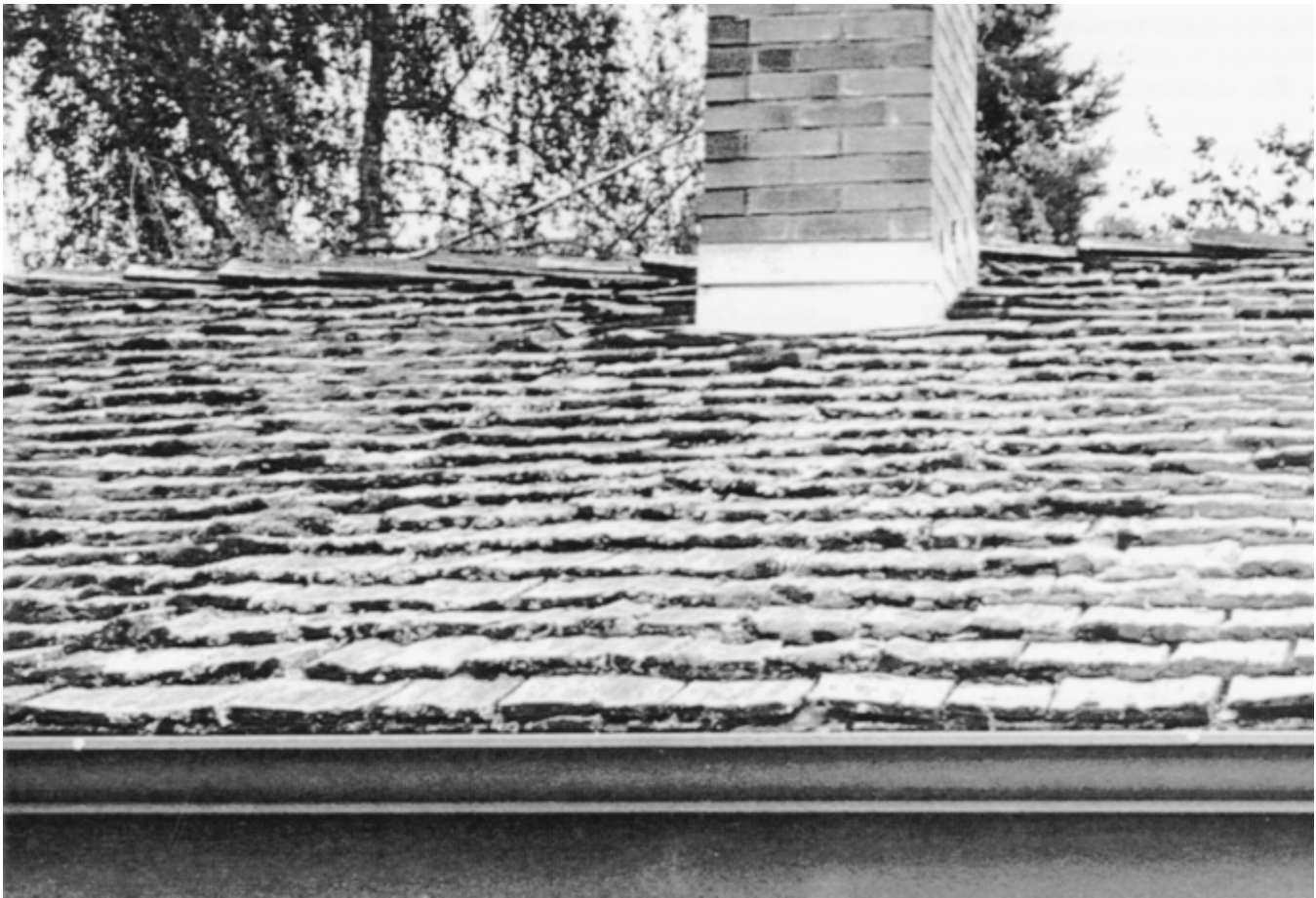
Figure 3.—Below this zinc chimney flashing, moss growth was inhibited, as indicated by the lighter colored roof surface. This leads some wood scientists to recommend using copper or zinc
