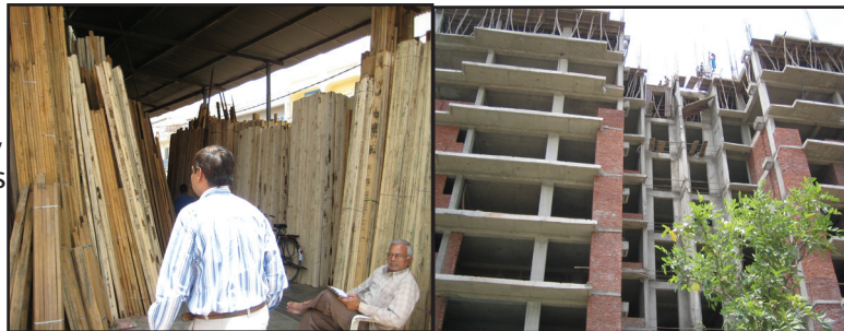
Typical retail outlet for shuttering (left) and shuttering used in construction of a multi-story concrete building (right).
