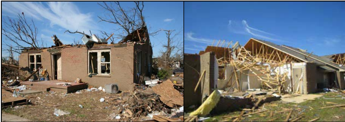
Typical damage observed to single family homes from tornado in Tuscaloosa, Alabama.
